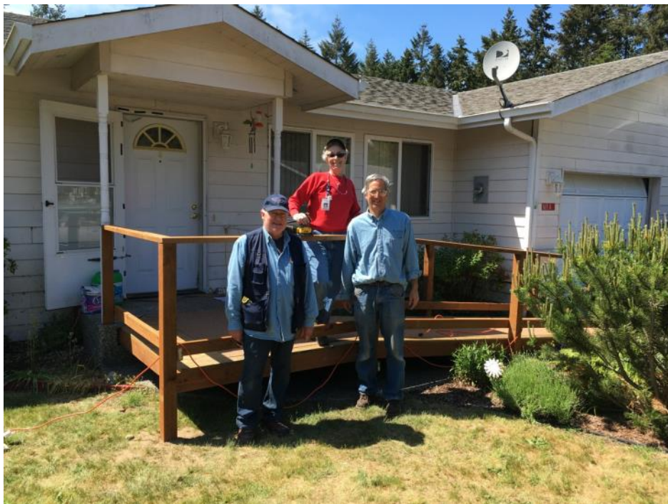
Completed ramp. David Parish, Jo Nieuwsma, and Todd Knoblock. Photos by Dan Nieuwsma, Michael Graham not shown.
